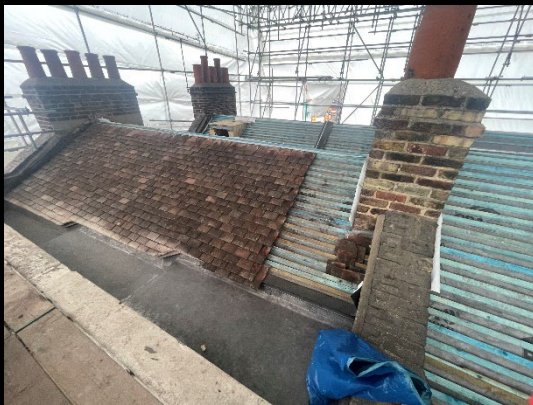
New roof gutters with strengthened roofs With the reinstatement of heritage roof tiles
